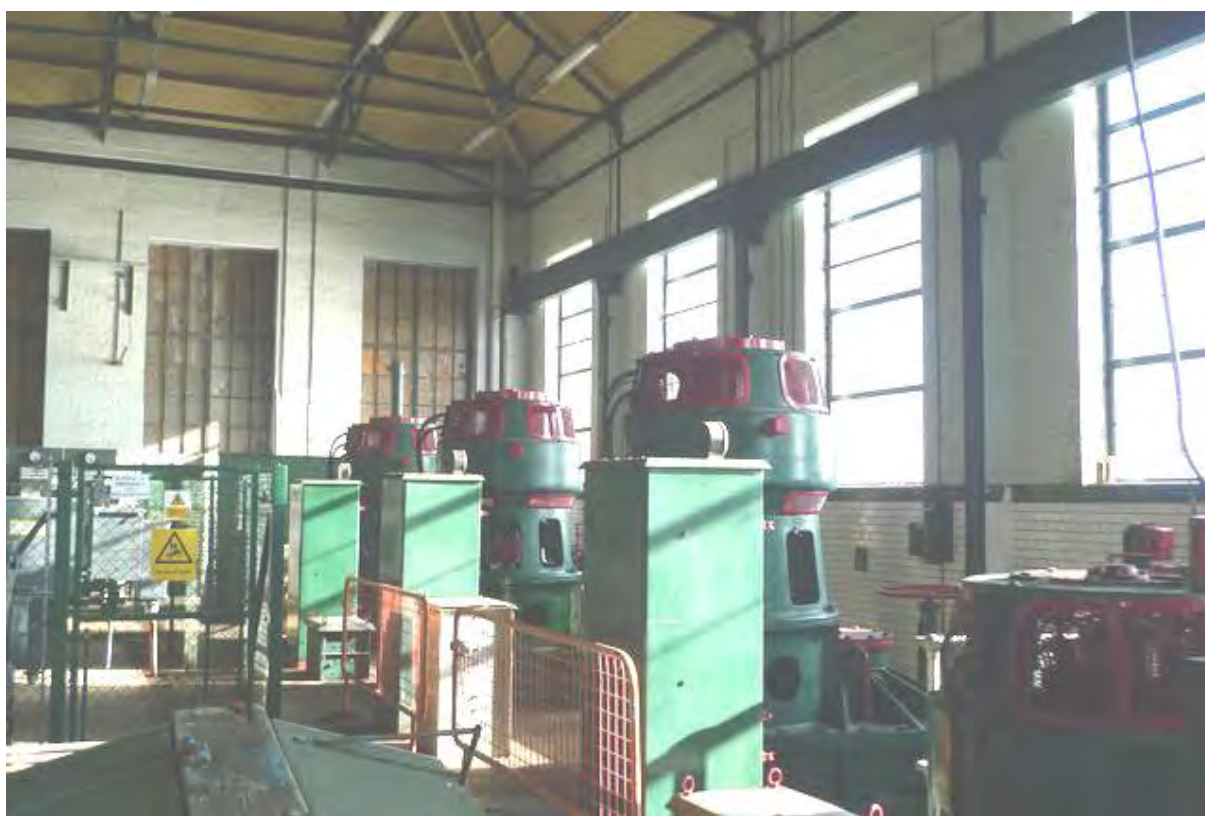
Figure 8.1: Mayflower Park Pumping Station
