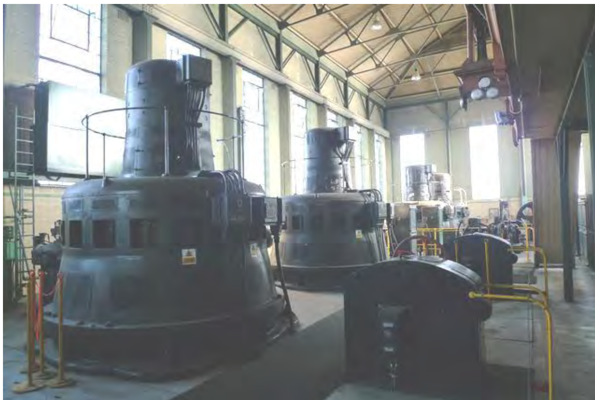
Figure 8.2: Pumping Station No.7 (King George V dock)
